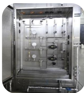
Multi-logistics switching system
